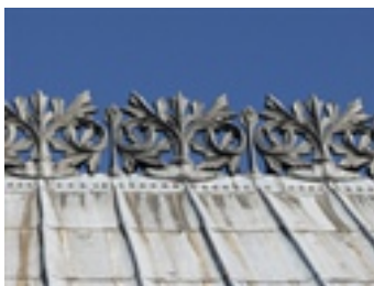
Lead roof of Notre-Dame de Paris, France, before the April 2019 fire. (credit: A. Timbert)
